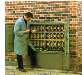
Cable distribution cabinet
